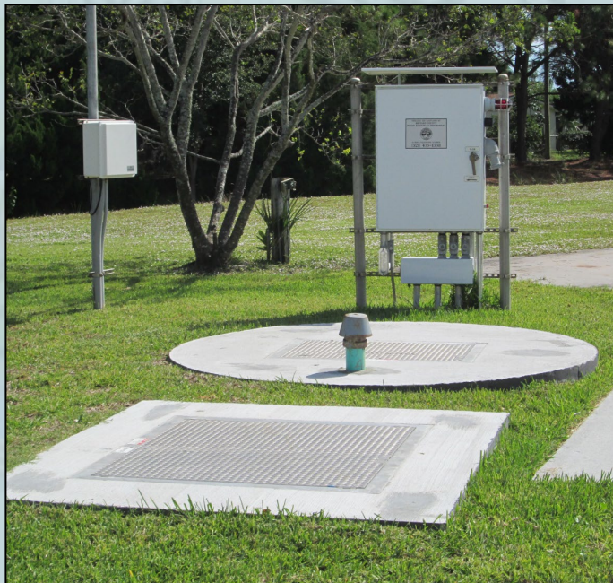
Figure 4 - Typical BCUSD Lift Station
